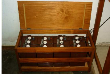
Figure 9. Battery pack in the HC of Shucusyacu.
