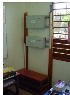
Figure 8. Server and battery loader in the HC of Shucusyacu
